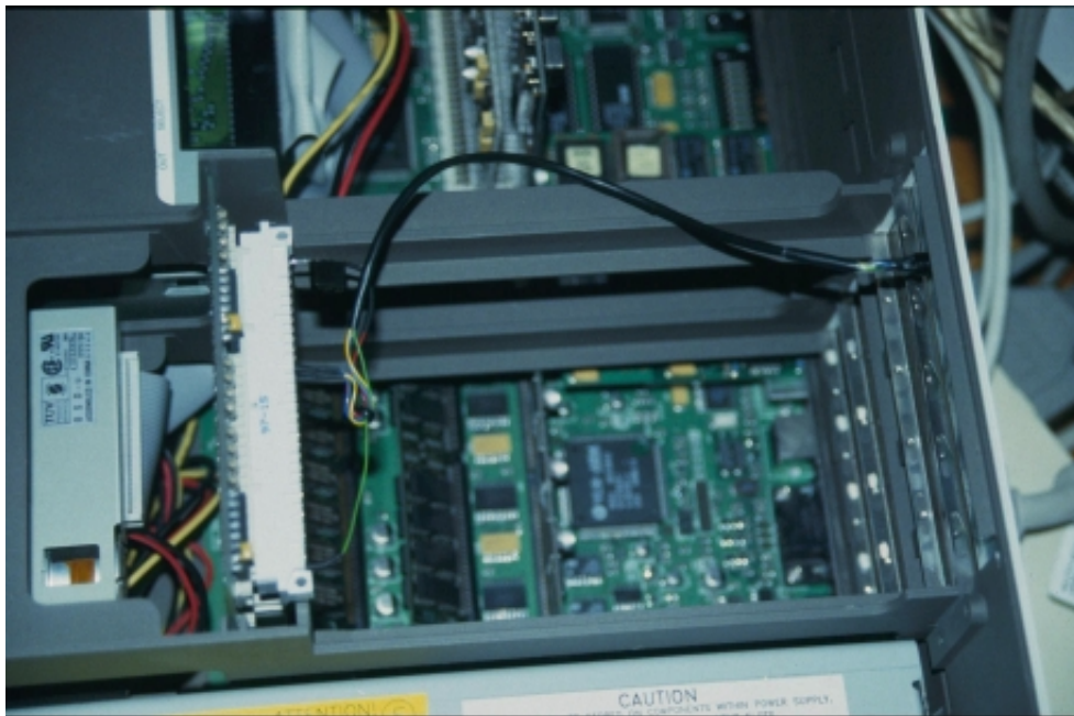
DIN41612 plug in place
